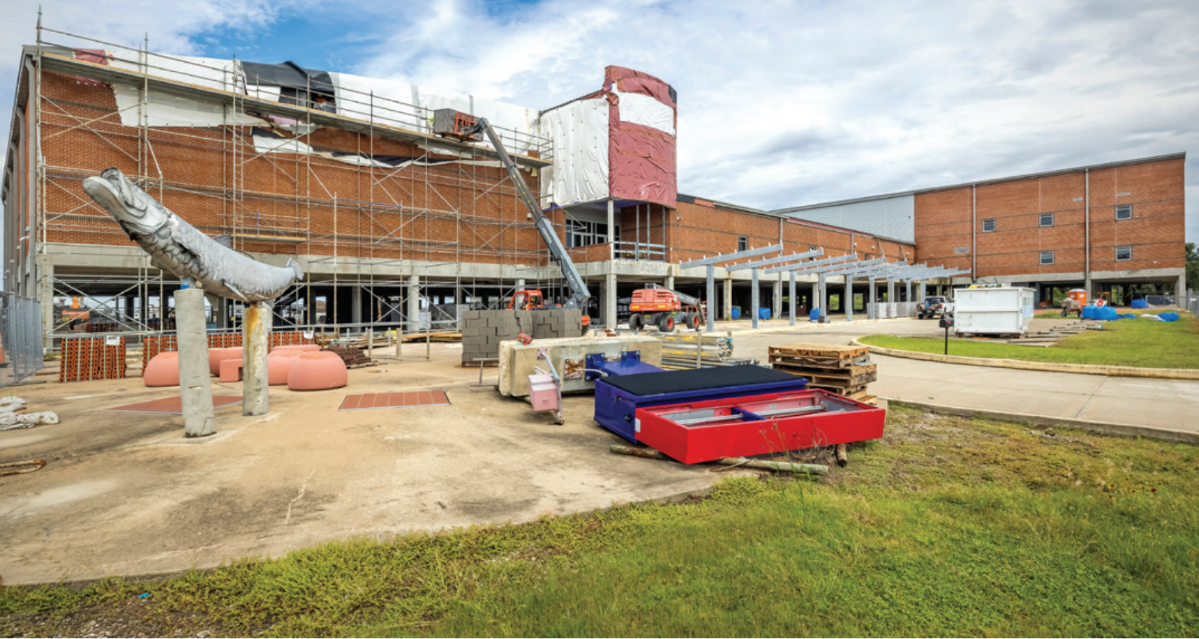
Construction workers continue repairs to South Cameron High School's main building following hurricanes Laura and Delta.
