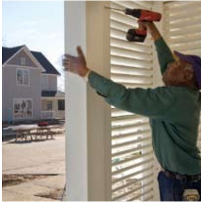
Workers put the finishing touches on affordable housing in Old South Baton Rouge—part of the federal HOPE VI grant issued in 2003.
