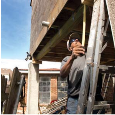
After gutting the flooded property, residents begin rebuilding a home in New Orleans.
